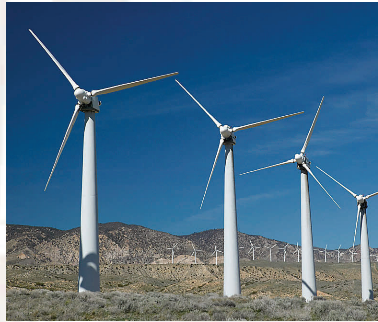
Typical Onshore Wind Farm
