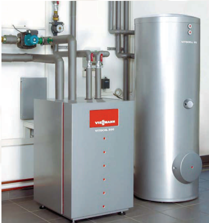
Viessmann Heat Pump Installation with Domestic HW cylinder
